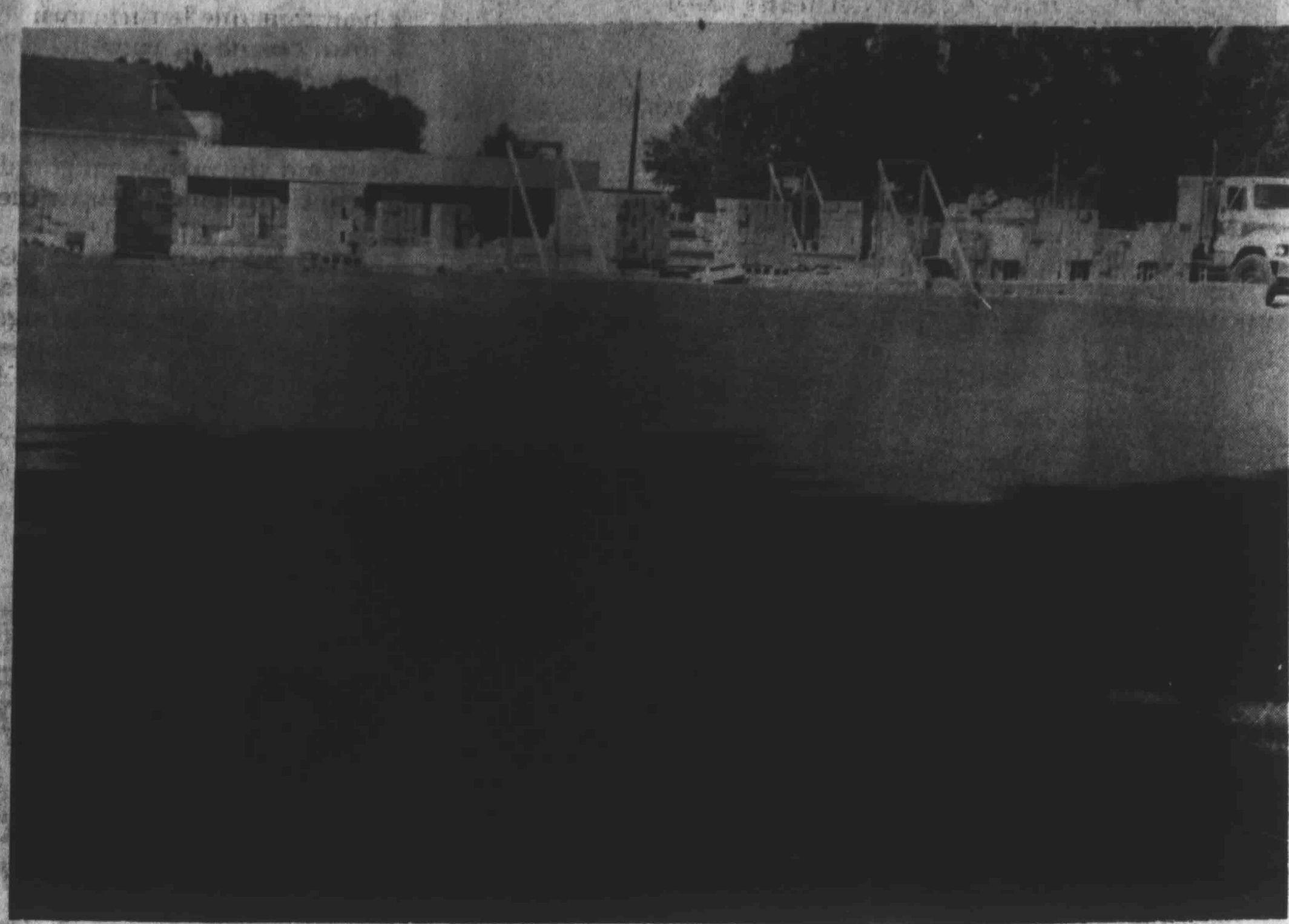
FIELD HOUSE at Halls High School is being built by Charles Seaton Construction Co., of Finley. The 50 x 100 ft. structure will contain visitor and home team dressing rooms, weight rooms, a coaches office, a laundry room, and a room for officials. Construction is expected to be finished by the end of September.
